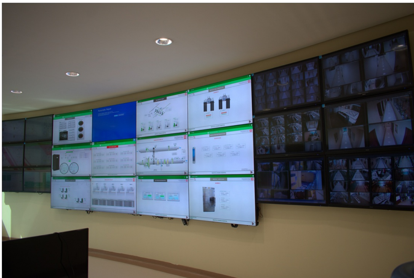
Figure 7. BMS and Integration Monitoring Screens
